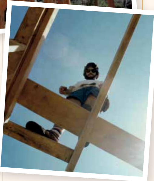
Above, left: Geoff Crane routing an exposed valley rafter, 1984; Bruce Giffin, roof framing, 1984. Facing page, above, right: Left to right: Derek Shue, Bruce Giffin, Geoff Crane, Eric Carlstedt. Below right: Riley Giffin and Bruce Giffin setting form boards, 1991; Geoff Crane, on the builder's level, and helper laying out a foundation, late '80s; Bruce Giffin and crew roof framing, 1988.
